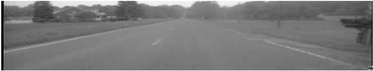
Right pavement markings indicated as “obscured”
