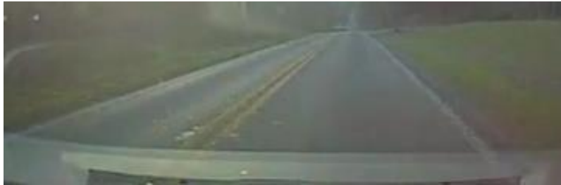
Pavement markings indicated as “visible”
