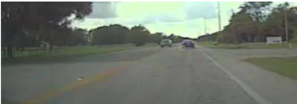
Pavement condition indicated as “moderate”
